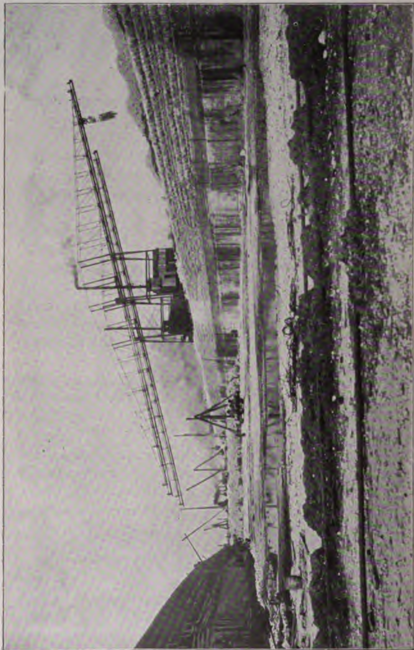
FIG. 13. A view of work on a big cut in the Chicago Sanitary and Ship Canal. The Chicago drainage canal was one of the most stupendous undertakings ever carried out by the city of Chicago. It provides for the disposition of Chicago sewage through an artificial canal from Lake Michigan through Chicago to the nearest point on the Illinois River at Lockport. See page 157.
