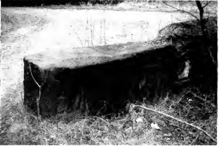
(a) MERSTHAM LIMWORKS. BASE OF STEAM ENGINE BUILT INTO WALL NEAR LIME COTTAGE.
